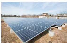
太陽光発電設備 Photovoltaic Facility
